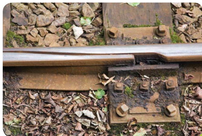
Figure 2 A breather switch. The sharp angle at which rails are cut ensures a relatively smooth and quiet ride for passengers.
